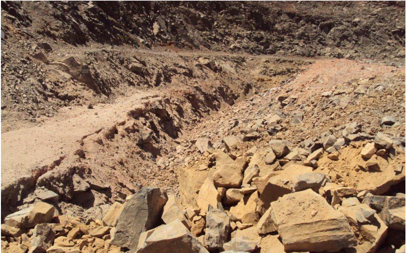
Photograph 4. Bottom of Butterfly pit looking west showing blasted material and the power trough out from a design berm.
