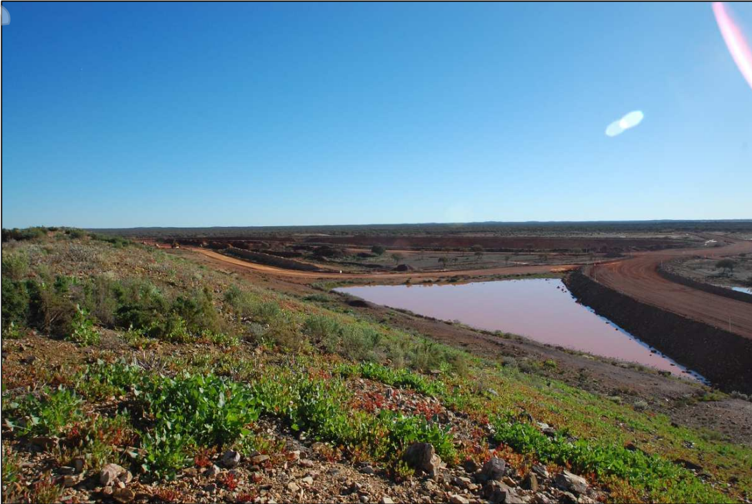
Photo 4. New haul road construction for ore and cyanide transport at the heap leach facility.
